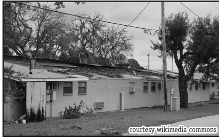
DESTRUCTION: Storm severely damage homes in Florida.
