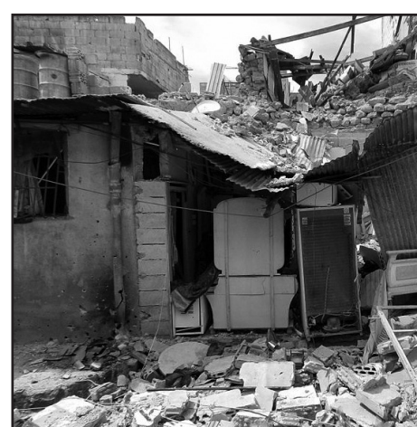
CRUMBLING TO THE GROUND: Buildings deteriorate and waste away.
